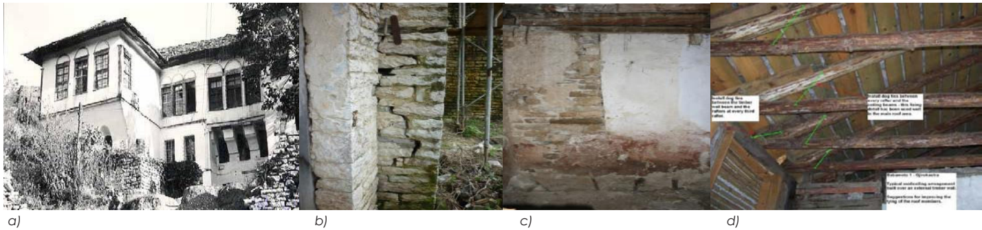
Figure 6: a), b), c), d): The Babameto's house before restoration, main damages of the house, the situation of the roof. Source: (CHWB, 2012).
