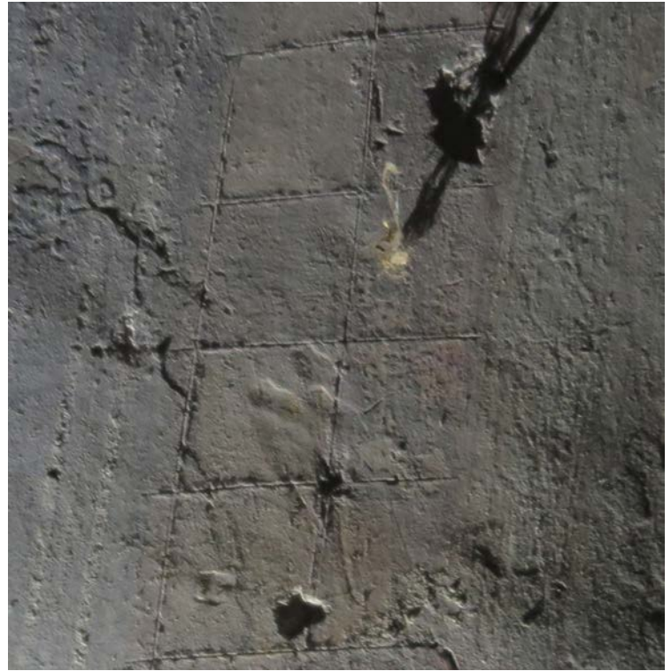
Figure 4. Preparatory scratching. Wall painting of the naos of St. Mary of Spile church. Source: Photo E. Çausi.
